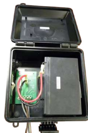
AA-BB128 (Internal View) AA128, Battery Box
